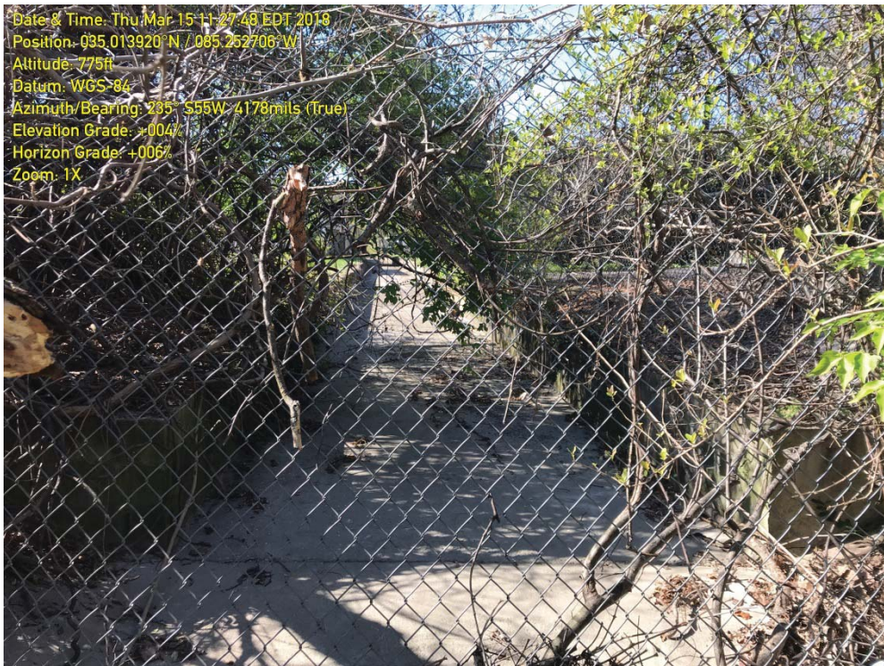
Photograph 4 – IMG_2717 - View of STR-1 looking upstream from near the culvert inlet at the edge of the existing ROW
