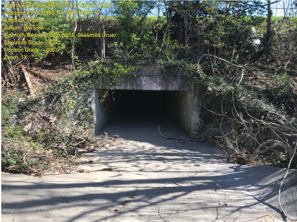
Photograph 5 – IMG_2718 - View of STR-1 looking downstream at the culvert inlet from near the edge of the existing ROW
