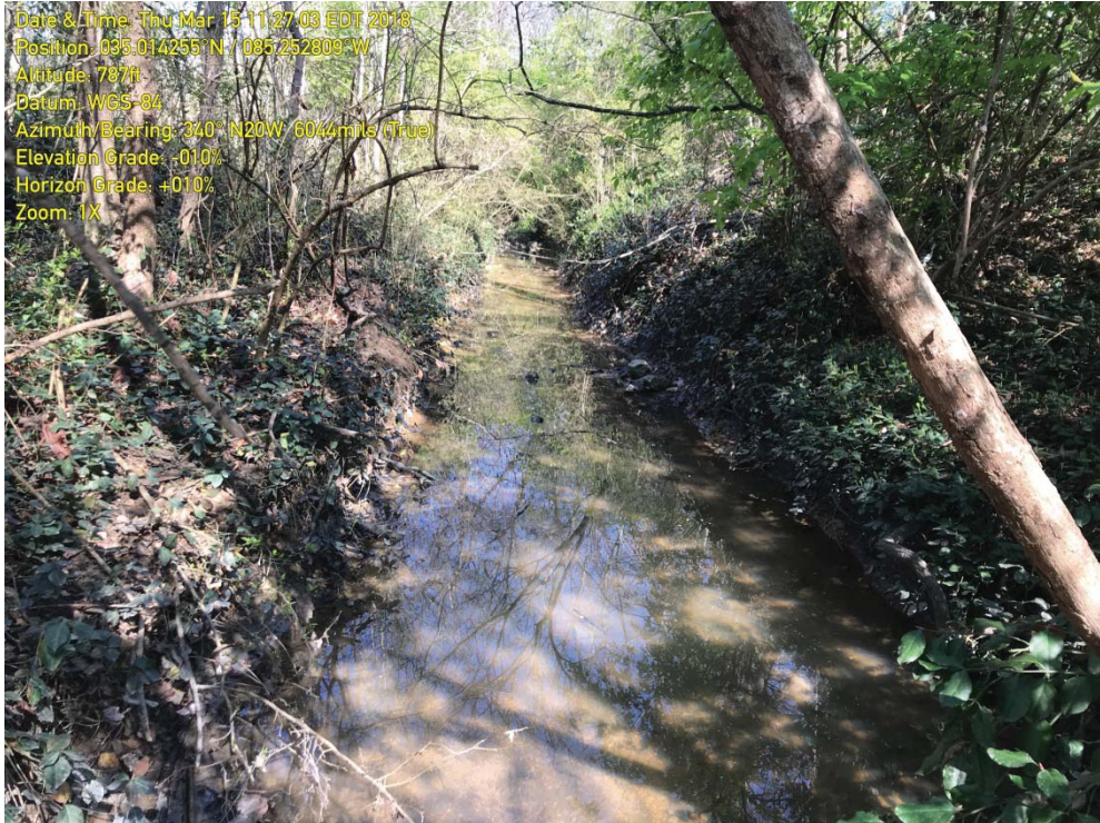
Photograph 7 – IMG_2715 - View of STR-3 looking upstream from the upstream end of the concrete channel shown in Photo 6
