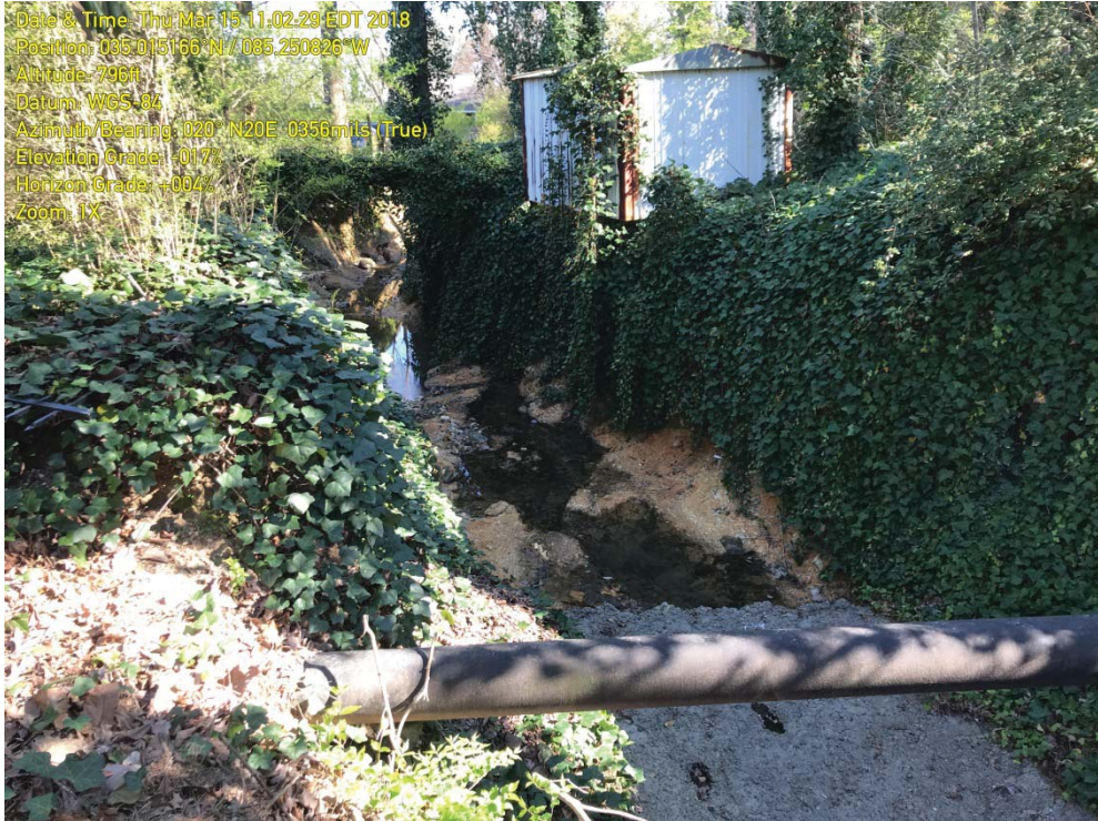
Photograph 3 – IMG_2710 - View of STR-1 looking downstream from the end of the gabion channelization
